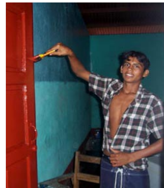
Thanks to CFUMC's support, the school at Los Playones, Nicaragua has started renovation inside the classroom. Shown above is painting being done in one of the classrooms that is being refurbished.
