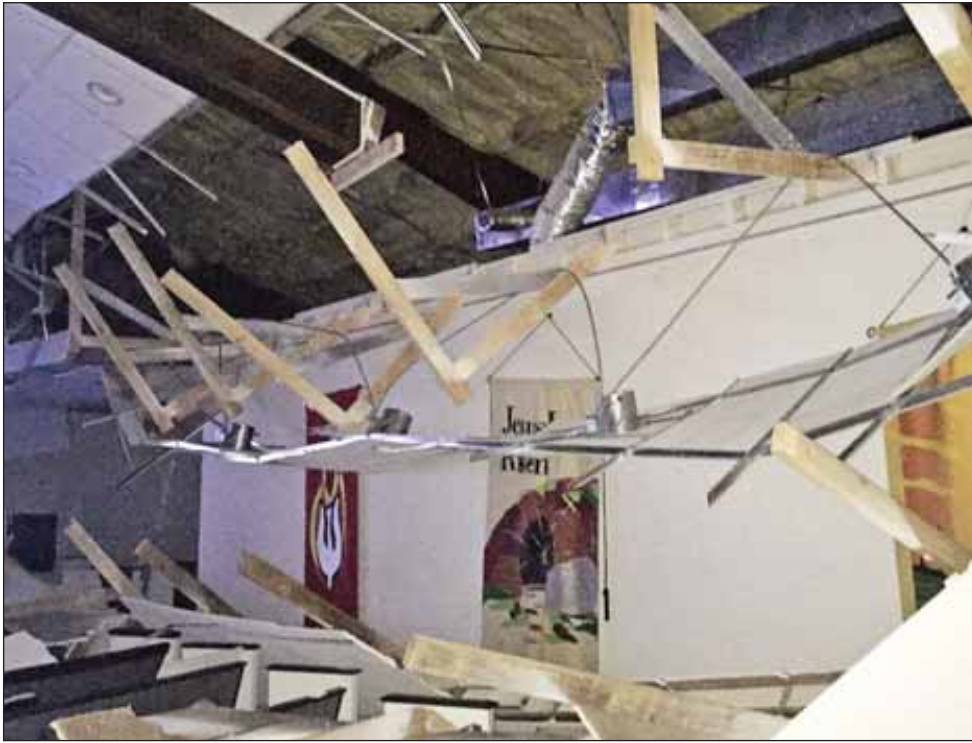
Hurricane Harvey caused extensive damage to the exterior and interior of Holy Cross Lutheran Church in Rockport.
