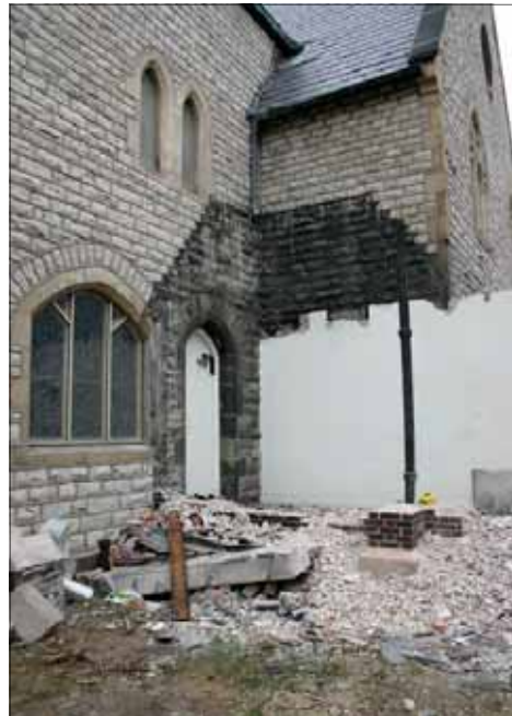
“Close up of entrance to the Chest Room. Note the dark discoloration of the limestone around the door. That’s due to heavy staining from a century of coal fires in industrial Detroit. The rest of the building was ‘cleaned’ in the early 1960’s (although not with good/appropriate technology).”
