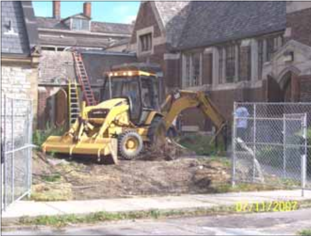
“Heavy equipment used to demolish the breezeway and concrete. What a job!”
