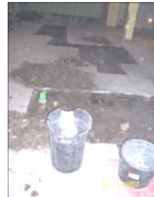
"A maze of subterranean water and sewerage pipes (some in poor condition) beneath the lower level."
