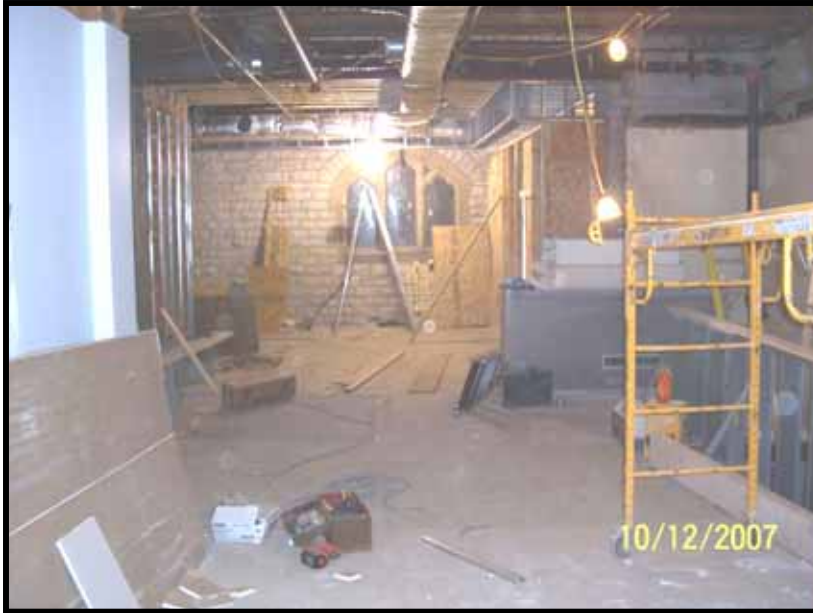
Looking from new nursery area toward St. Michael's Chapel where a new door will be constructed.
