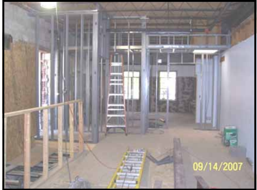
Looking east toward new nursery, wall skeletons, door on left to Sibley and steps to lower level
