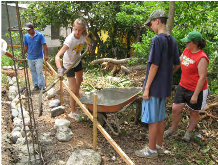
Christa Eberhard and Collin Ray shovel concrete for a new home's foundation in Quimistan
