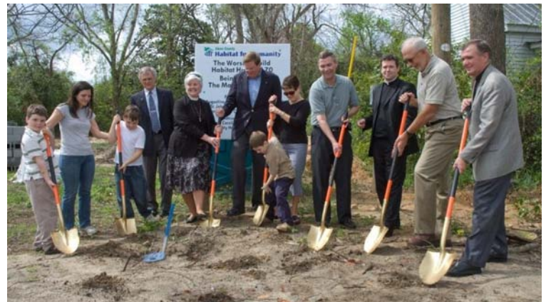
Pastors from four churches join Habitat's Richard Church and the Matthews family for "The Worship Build" groundbreaking ceremony.
