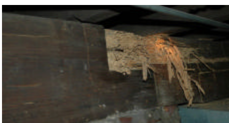
Deterioration of beam underneath south transept
