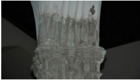
Chemical peel of column showing wood structure
