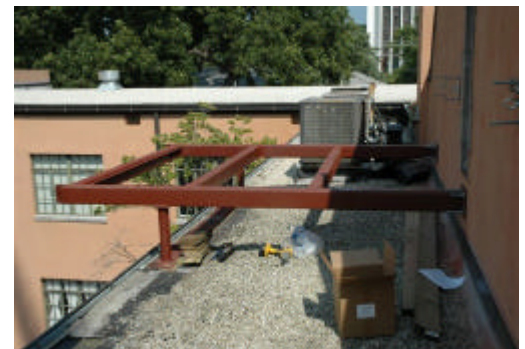
Location of one of chillers
