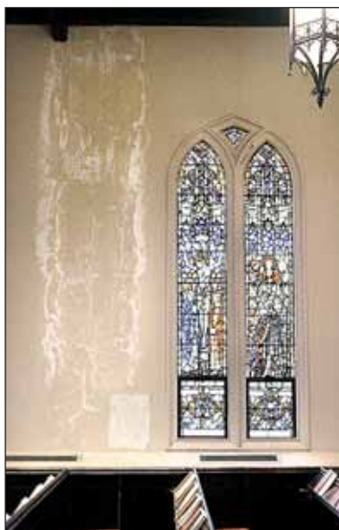
Water damage from a deteriorating roof is a large problem in the sanctuary.
