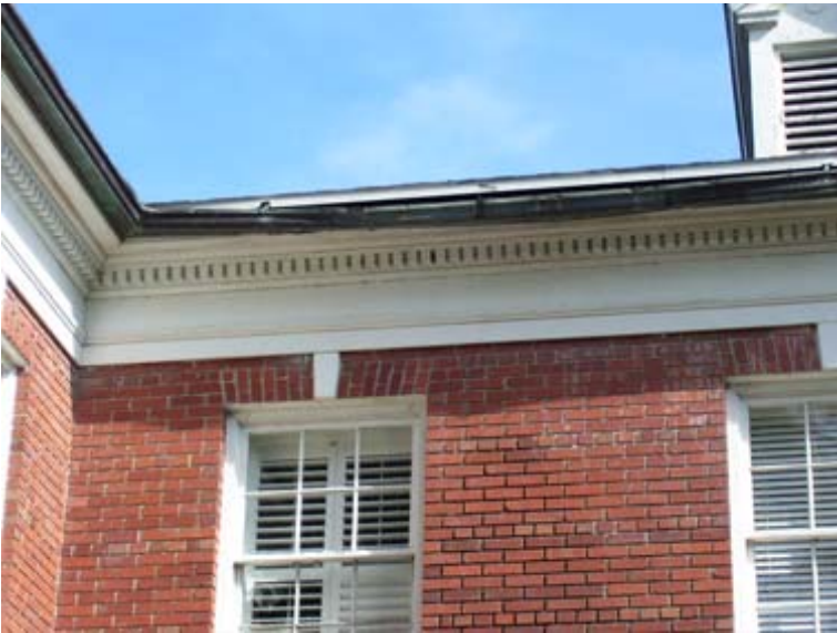
Gutters above the New England Avenue portico dangle and are ineffective.
