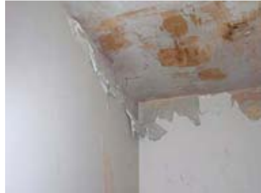
Damage from wind-driven water from 2004 hurricanes.
