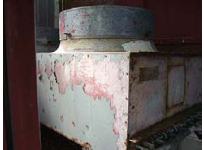
Current Outside Unit near the Kitchen
