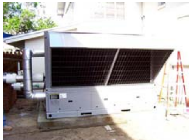
New Chiller Unit serving the Education Building
