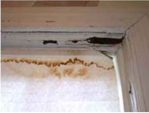
Rotted interior window in the second floor lobby bathroom that needs immediate replacement.
