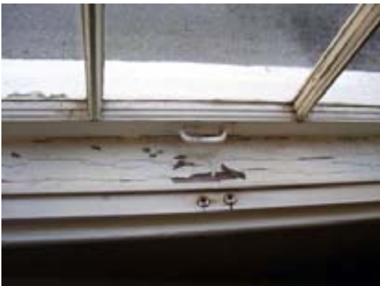
Deteriorating, chipped paint invites more extensive and costly repairs!
