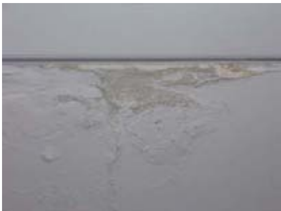
Wind-driven water damaged the paint and plaster below the windows in our Sanctuary.
